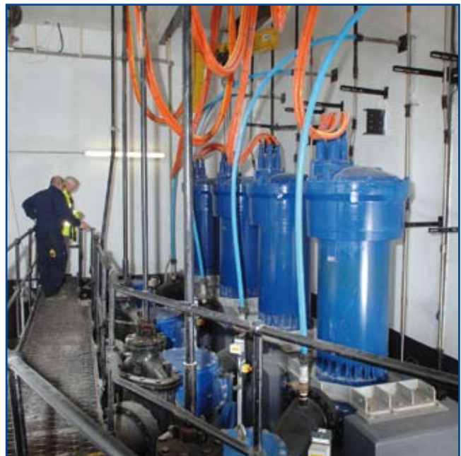
A typical flywheel installation, pumping raw sewage. 4 x Immersible pumps with 175KW motors and a duty of 300l/s at 35m head per pump.
